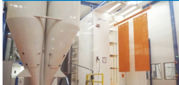
Fully automated state-of-the-art paint plant
