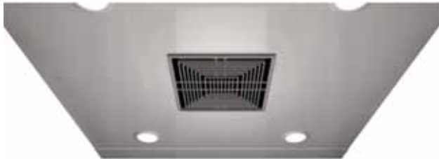
CT002 Finishes : Painted; Stainless Steel Lighting: CFL; LED Ventilation: Axial Flow fan (strong air flow)
